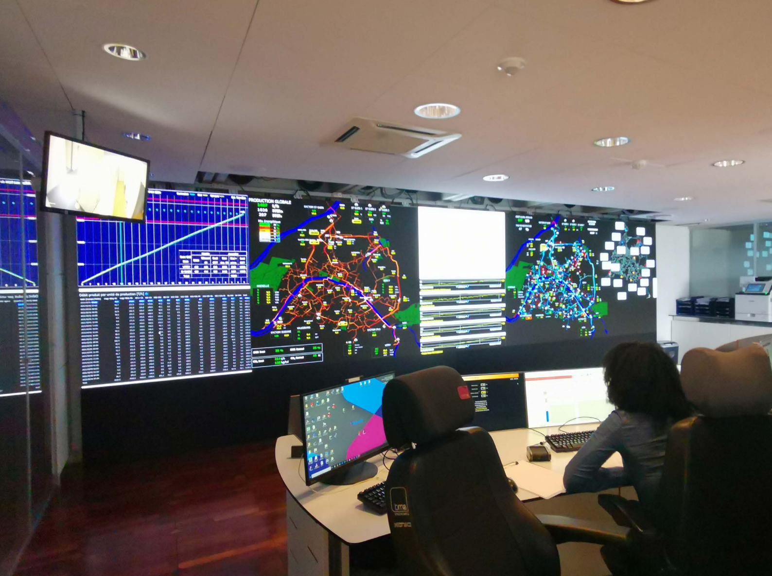
Water Management Control Room — Paris, France 13x5 TVF-1.2 + netPIX
