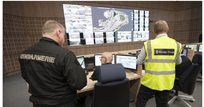
Eurotunnel Control Room Calais
